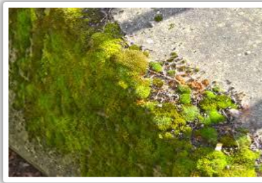
Layer of Moss on Wall
